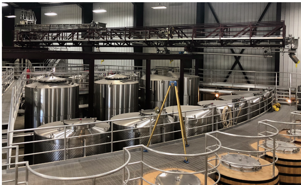
An incline, cleated conveyor carries pomace to a membrane press (above) and a large rotating arm with a conveyor carries destemmed and sorted grapes to the top hatches of tanks at the older facility.
